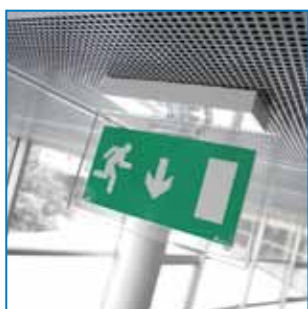
Planete60, ceiling application
