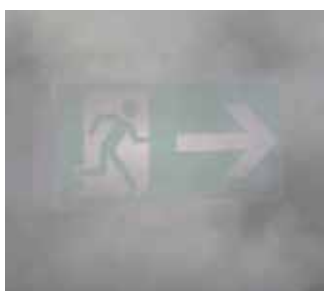
Badly illuminated escape sign
